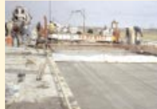
All U.S. states have used silica fume at least once in bridge deck applications.
